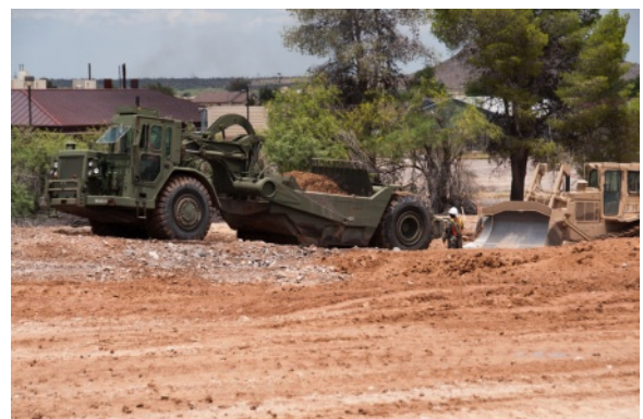
Members of the 258th Engineer Company clear land adjacent to Florence High School during an annual training event June 1-12. The work completed by the 258th is the beginning of a project to build practice fields for student athletes from the high school. (U.S. Army National Guard Photo by Spc. Wes Parrell)
