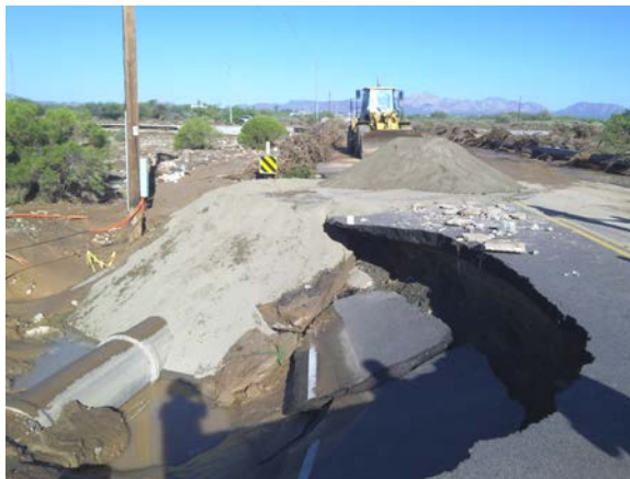
The Centennial bridge in La Paz County received major damage during the September 2014 storms. (Photo by ADEM Recovery)
