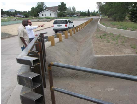
Dustin Woodman, Engineering Division Manager at the Coconino County Department of Public Works, explains to ADEM Mitigation Grants Program Manager LaMar Brown how federal grant funds were used to build floodwater conveyances in the community of Timberline. Since the Schultz Fire in 2010, the area has experienced over 60 post-fire floods.
