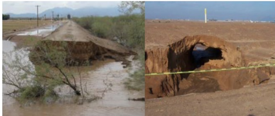
Non-levee embankment failures in Pinal County Source: Pinal County MJHMP, 2015
