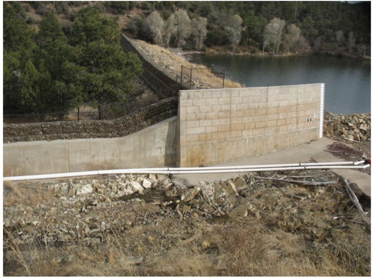
Lynx Lake Dam and emergency spillway showing recent dam safety mitigation measures to raise the dam crest. Source: JE Fuller, 2009
