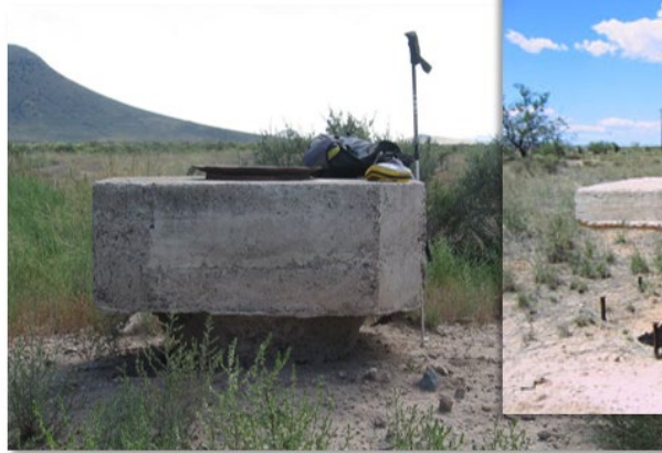
Subsidence at well casings Source: AZGS
