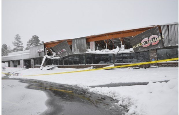
Roof damage from January 2010 snow storm in Flagstaff, AZ Source: Betsy Bruner, AZ Daily Sun
