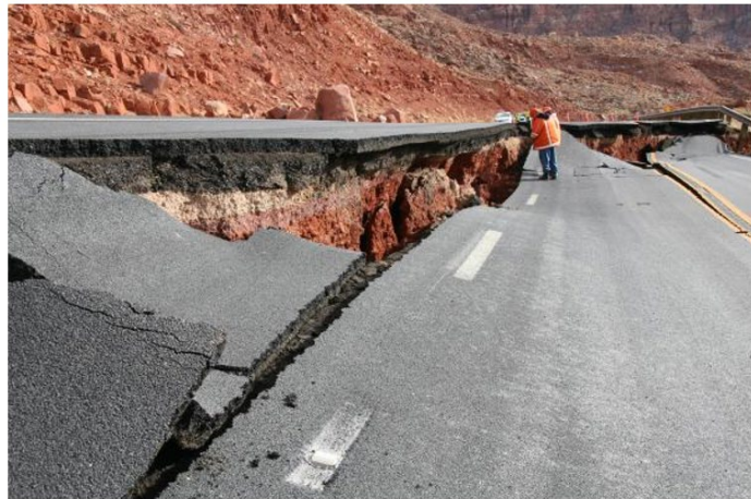
Landslide damage to US 89 at Echo Cliffs near Page, AZ Source: AzDEMA, 2013
