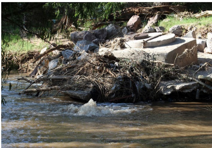
Nogales Wash – International Outfall Interceptor rupture at manhole location in Nogales, AZ Source: AZ Governor's Office, 2017
