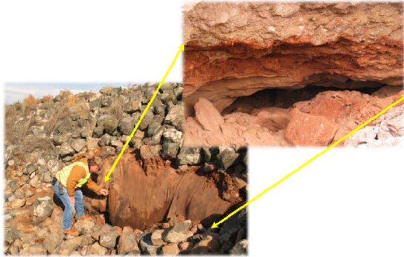
2004 Winslow Levee Piping Failure – Landslide photos Source: USACE, 2016
